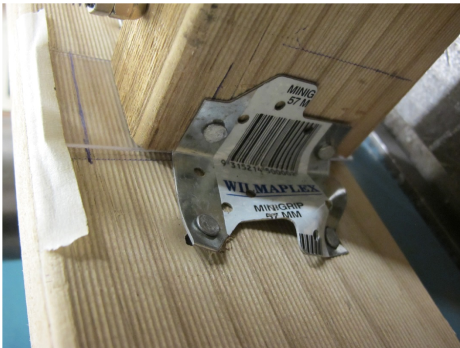
Figure 7 Typical failure of Mini grips, buckling of Mini Grip steel and bending of nails.
